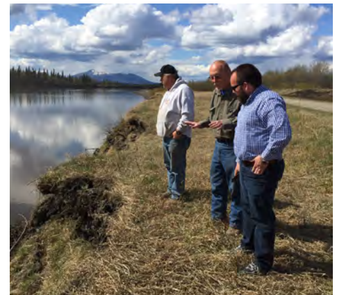
DOT&PF staff and McGrath leaders viewing erosion problems at McGrath airport
