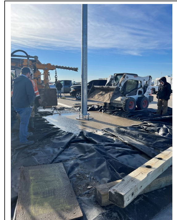
Photo: Test site construction at UNL for Light Pole Foundation Embedment project.
