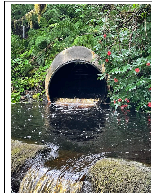
Photo: Slip lined culvert at 9-mile Creek in Juneau, AK where fish pass trials were conducted.
