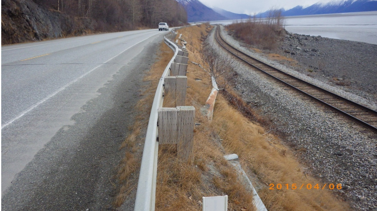
Exhibit 3. Retaining wall in Poor condition, Seward Highway. The wall is bowed outward, causing deformation of the guardrail and pavement.
