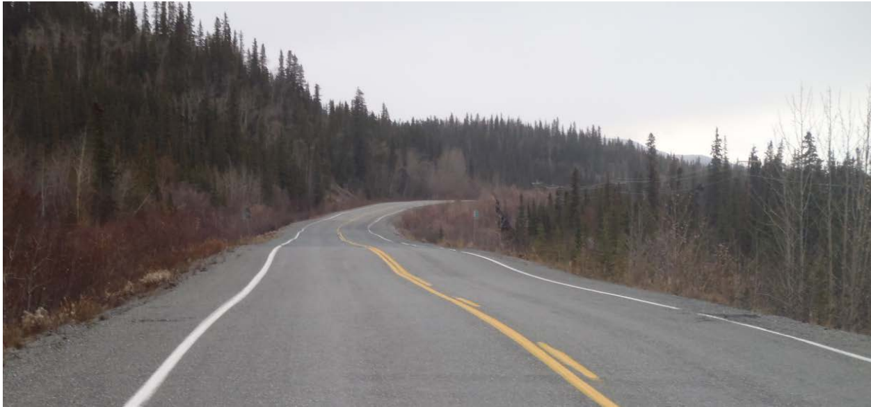
Exhibit 2. Soil slope in Poor condition, Tok Highway. Movement is relatively rapid, necessitating frequent maintenance to keep the road passable.
