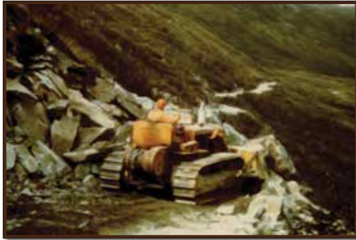
Clearing a rock-slide on Williamsport-Pile Bay Road with a bulldozer. Carl and Lyle Williams
