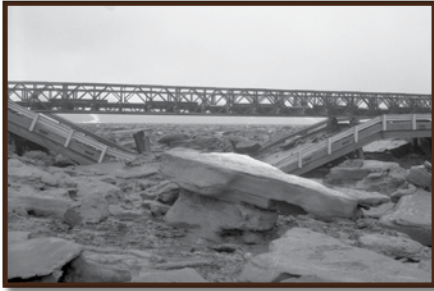
Earthquake damage to the Seward Highway bridge over Twentymile River near Portage on Turnagain Arm, following the earthquake of March 27, 1964.
