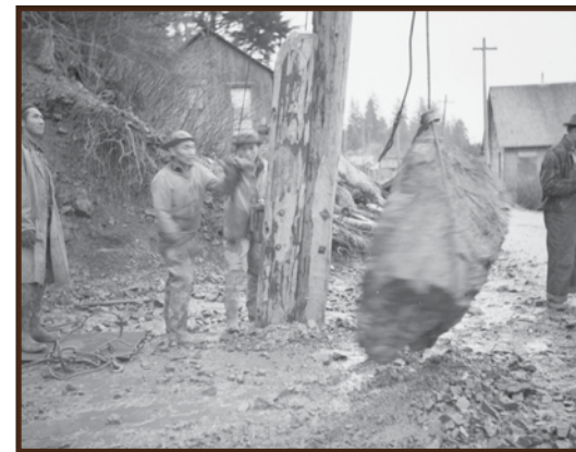
Men employed by the Civilian Conservation Corps working on a breakwater near Kake, 1941.
