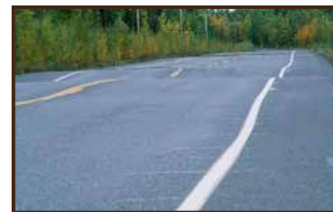
Frost heaves on the Richardson Highway.
