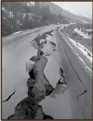
A crack on the Seward Highway caused by the earthquake.
