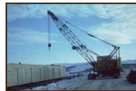
Removing the barracks at the Old Man camp on the Haul Road (now Dalton Highway) during the construction of the Trans-Alaska Pipeline, February 1976. Many of the camps were modular to allow for easy movement along the construction route.
